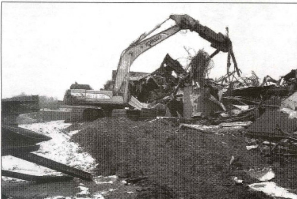
E. Luke Greene Co's Allied Gator Multi Tool (MTR70) mounted on a Kobelco 300, shears steel scrap to manageable lengths at the former Beacon Manufacturing Plant near Asheville, NC.
