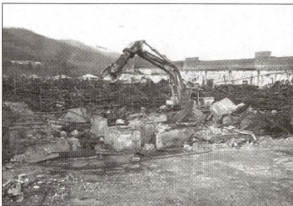
The September 2003 fire leveled most of the over one million sq. ft. former textile plant and was considered to be one of the largest manufacturing fires in North Carolina history. As a result, the debris needed to be cleared.
