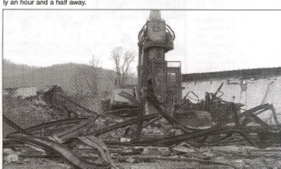
Depending on the material that needs to be removed or processed, the company uses either of the MTR70's two interchangeable jaw sets. On steel structures, the MTR70 shear jaw is used as a primary tool to cut steel beams.
