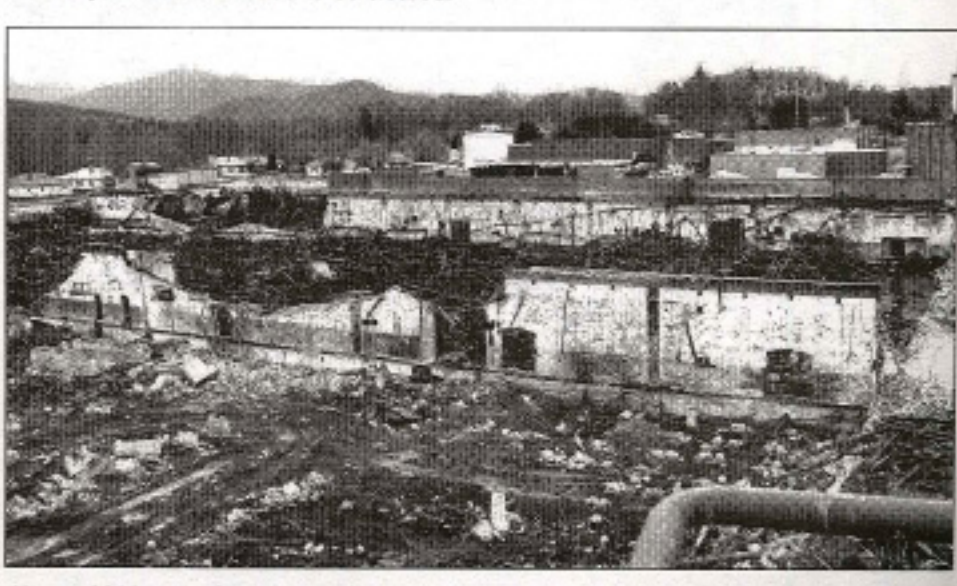
Almost 6000 tons of steel was recycled and over 57,000 tons of contaminated debris was transported to Palmetto Landfill in Spartanburg, SC, as a result of the September 2003 fire.
