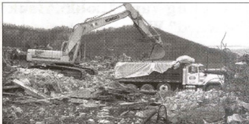
In all, the company hauled nearly 3,800 truckloads of asbestos-contaminated C&D waste material from Asheville to a waste management facility in Spartanburg, SC, which is nearly an hour and a half away.
