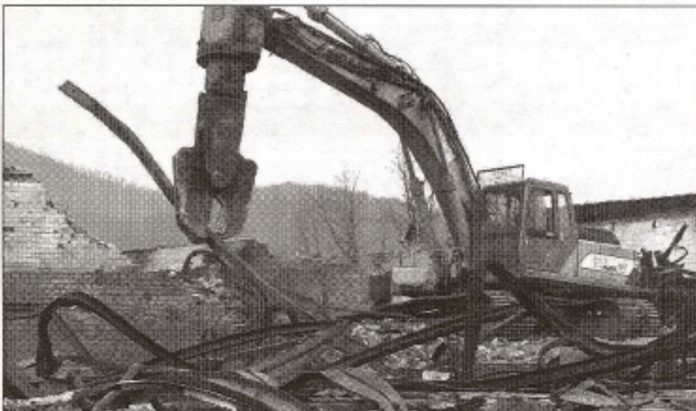
The Allied-Gator MTR70 is frequently used on demolition jobs that require the company to remove steel and concrete buildings. The MT series Multi-Tool is used to tear through the material within a structure, removing large pieces one at a time and later, reducing the steel and concrete to smaller-sized pieces for ease of transportation.
