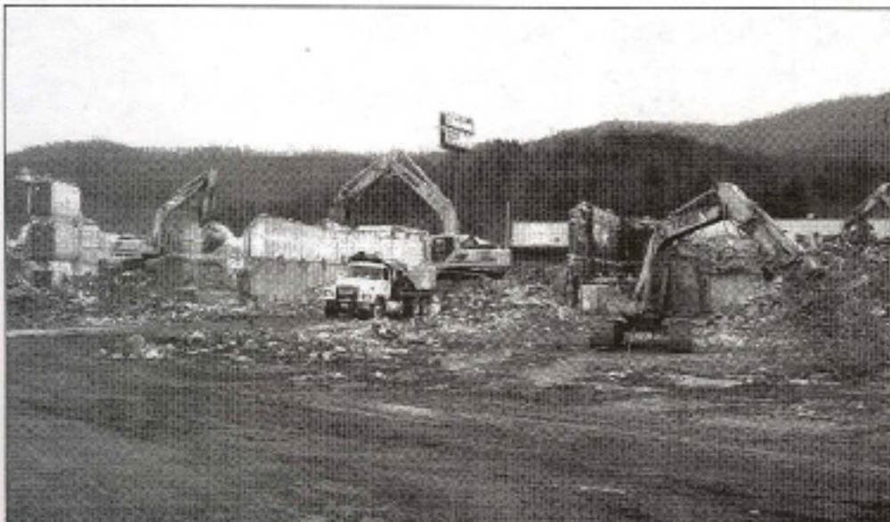
Within the company's fleet are seven Kobelco excavators - here they are working in tandem to process the materials.
